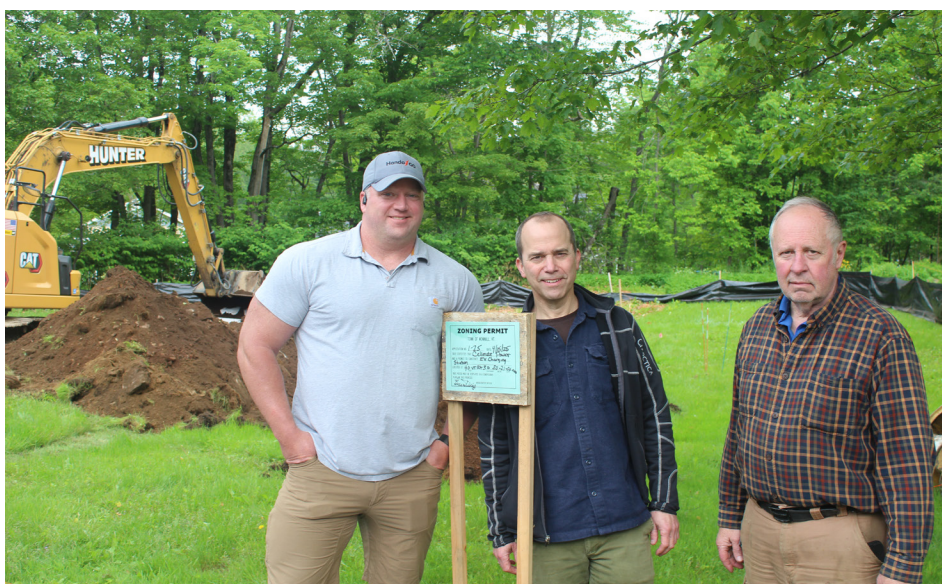
Erik Moses (Center) stands with Stuart Coleman (Right) and Tyler Thompson (Left) during the construction process
